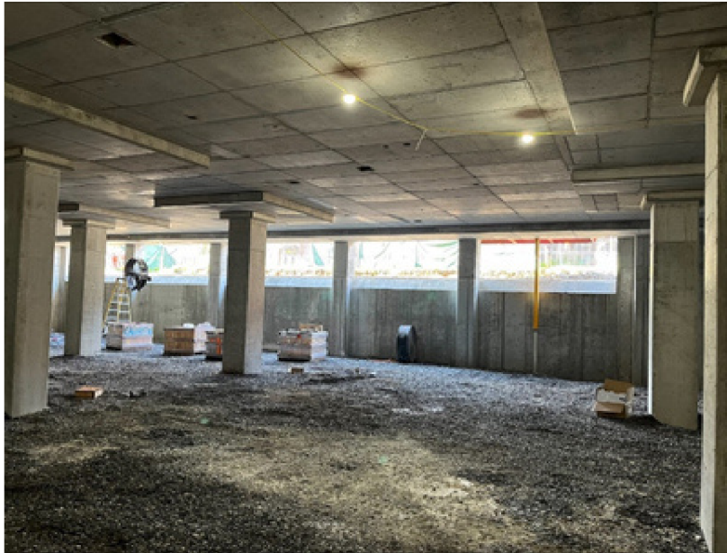
View of the basement where windows let in a lot of light.
