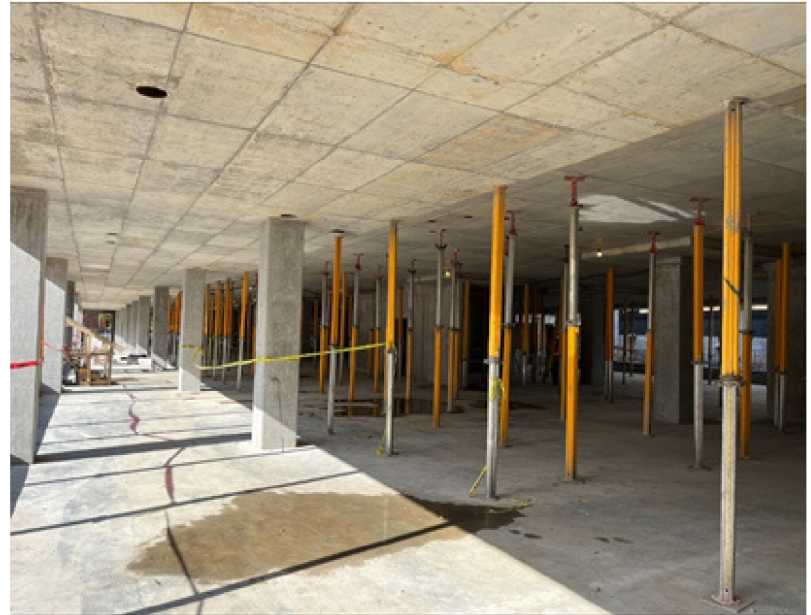
View of the main floor. Metal supports have to stay in place until the concrete is completely dry.
