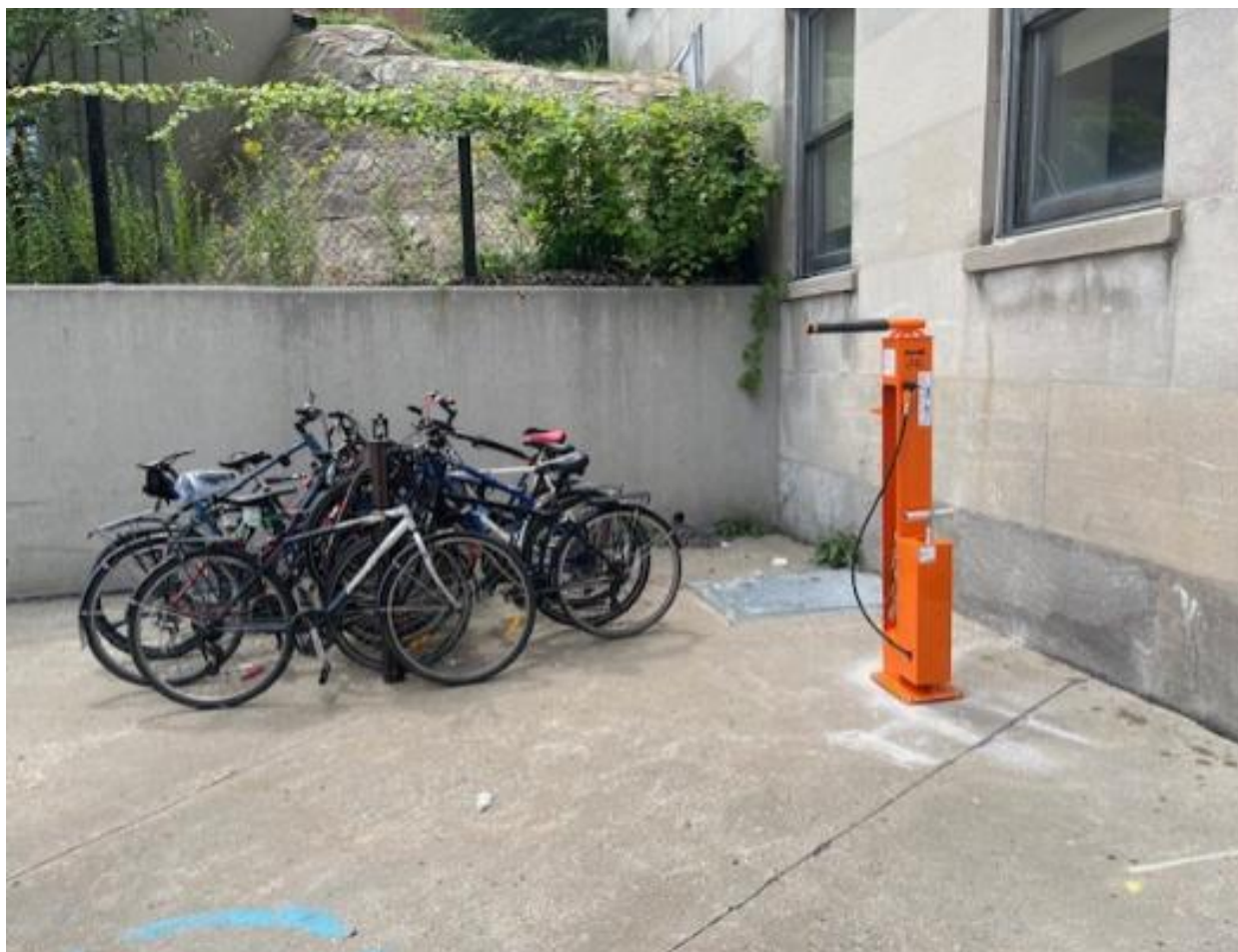
One of the bike repair stations installed at our sites. It allows cyclists to carry out minor repairs on their bikes at the workplace.
